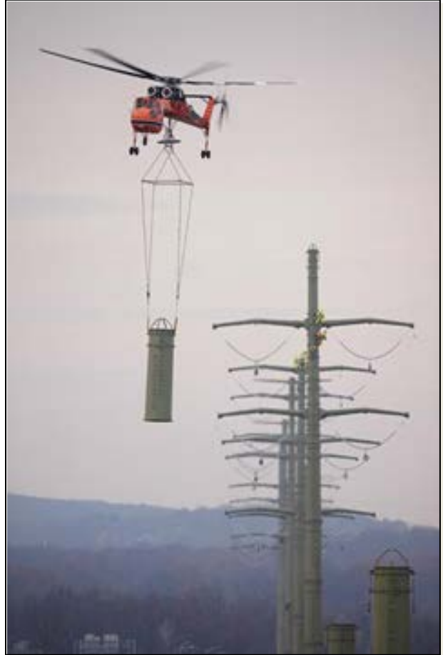
Susquehanna Roseland Project
