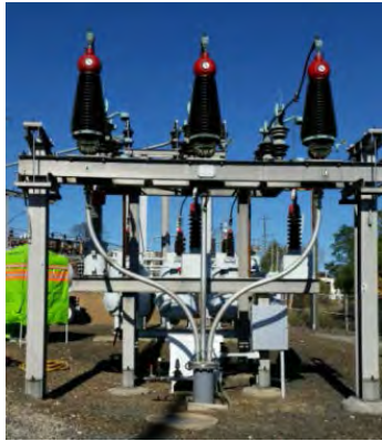
Figure 4– HPFF Termination (provided by PECO)
