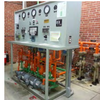
Figure 7- Pumping Plant (provided by BGE)
