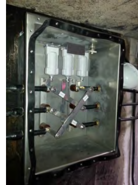
Figure 6- Link Box (provided by PECO)
