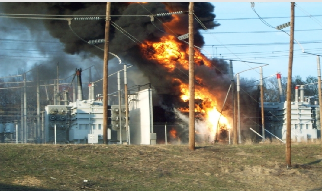
500 kV Transformer Failure in 2000
