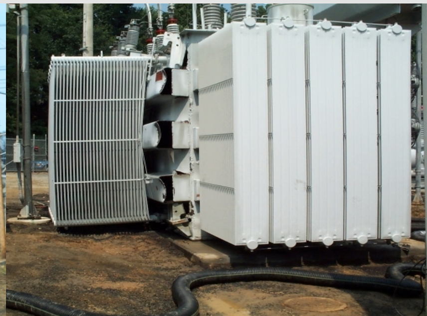
230 kV Transformer Failure in 2001
