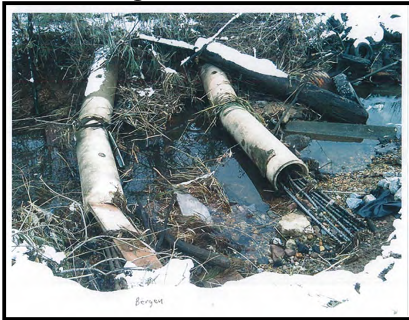
Existing Control Cables
